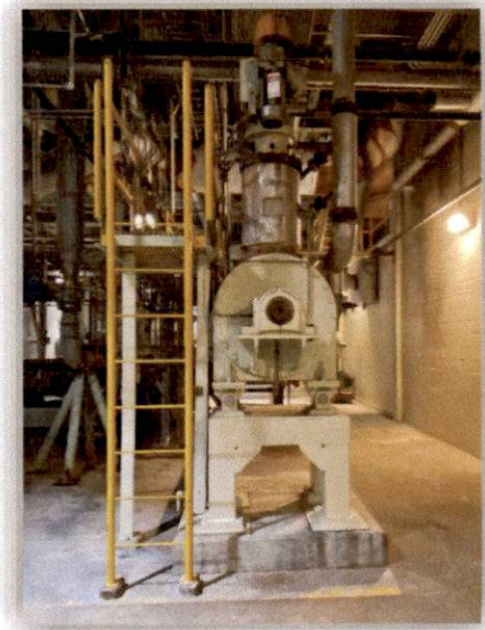
Preheater (side view)
