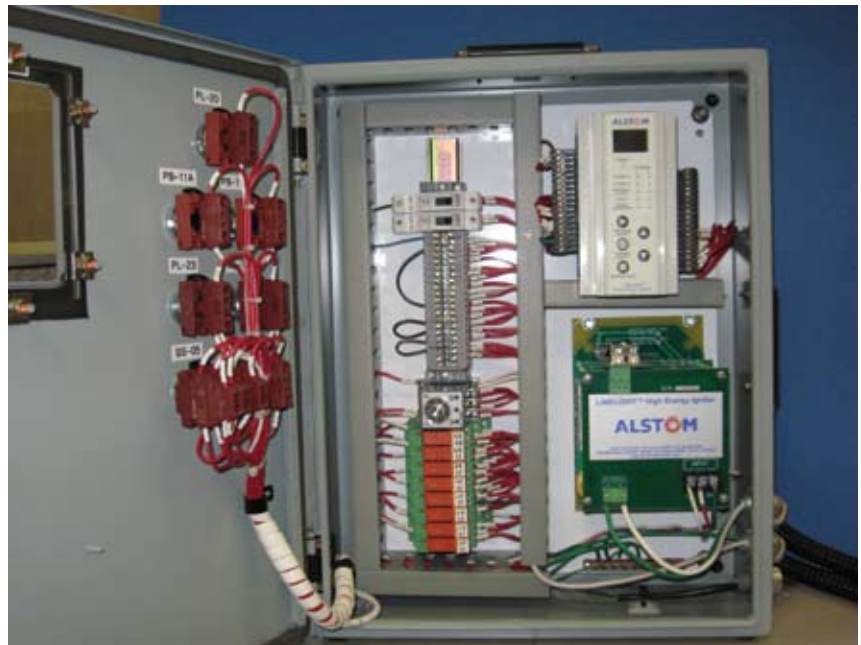
Ignitor Control Cabinet shown with Flame Signal Analyzer installed
